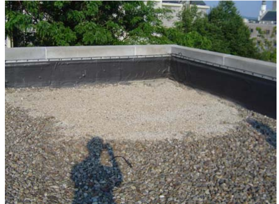
Classic patch location in the southeast corner of a large flat roof. Fractured peastone on top of large stone ballast.
