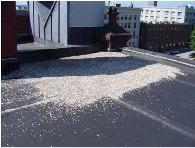
Fracture peastone patch on the southwest corner of a roof with low parapets and adjacent to another roof. Note large structures that may provide too much shade.
