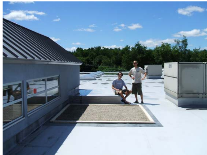
Rounded peastone patch with a frame and landscape fabric, adjacent to a taller section of the building. The wall provides shade but may be too tall.
