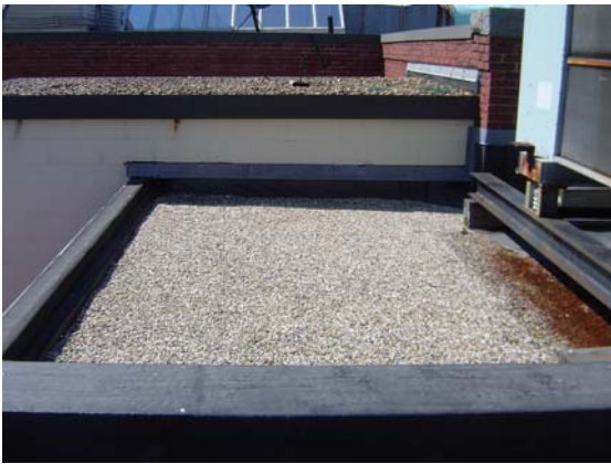
Fractured peastone patch in a small section on the southeast side of a larger roof, but adjacent to another building roof. Note shade from AC unit on right.
