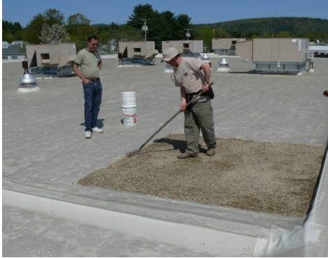
Installing a gravel parch at Keene Cinemas in 2008. Photo by Ken Klapper.
