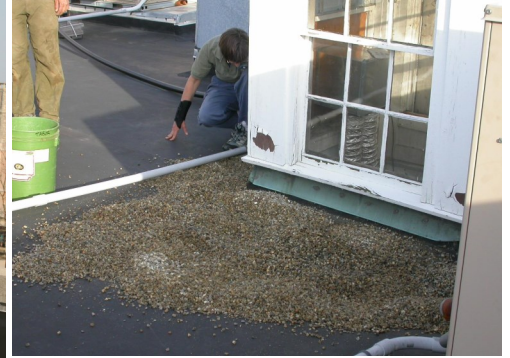
Installing a gravel patch at Salloway & Hollis in 2007. Photo by Stephanie Parkinson.
