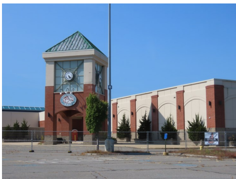
The Steeplegate Mall fenced off in August 2024 preparing for demolition. Photo by Rebecca Suomala.
